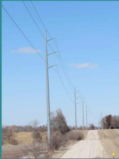
Typical 161kV Vertical Transmission Pole
